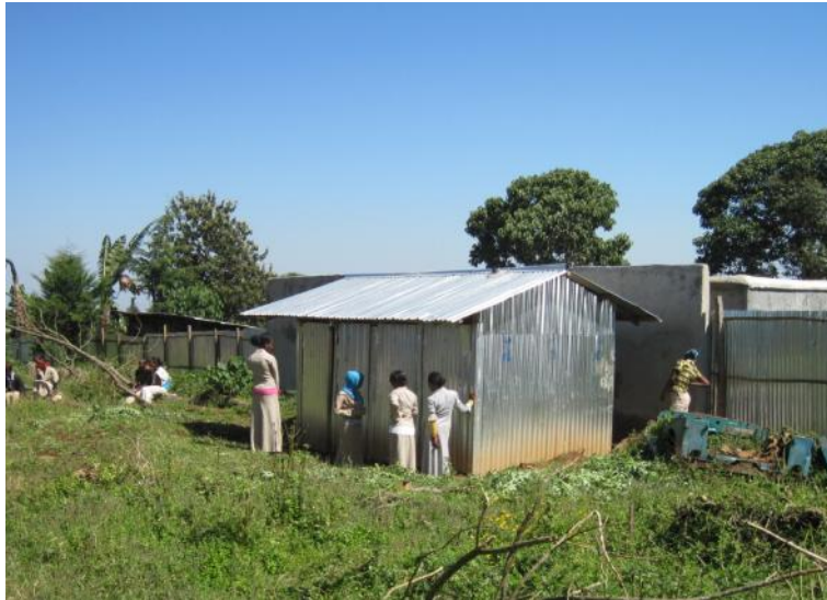
New Girls' Toilets at Nekemte Preparatory School funded with £1000 from the Estepona-Ethiopia Link
